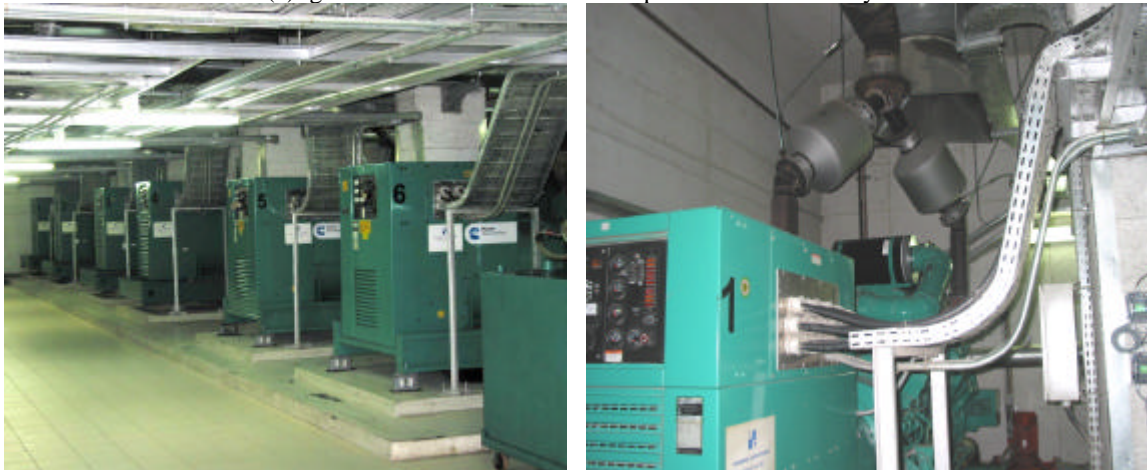
(c): The six Onan generators at the Movenpick
